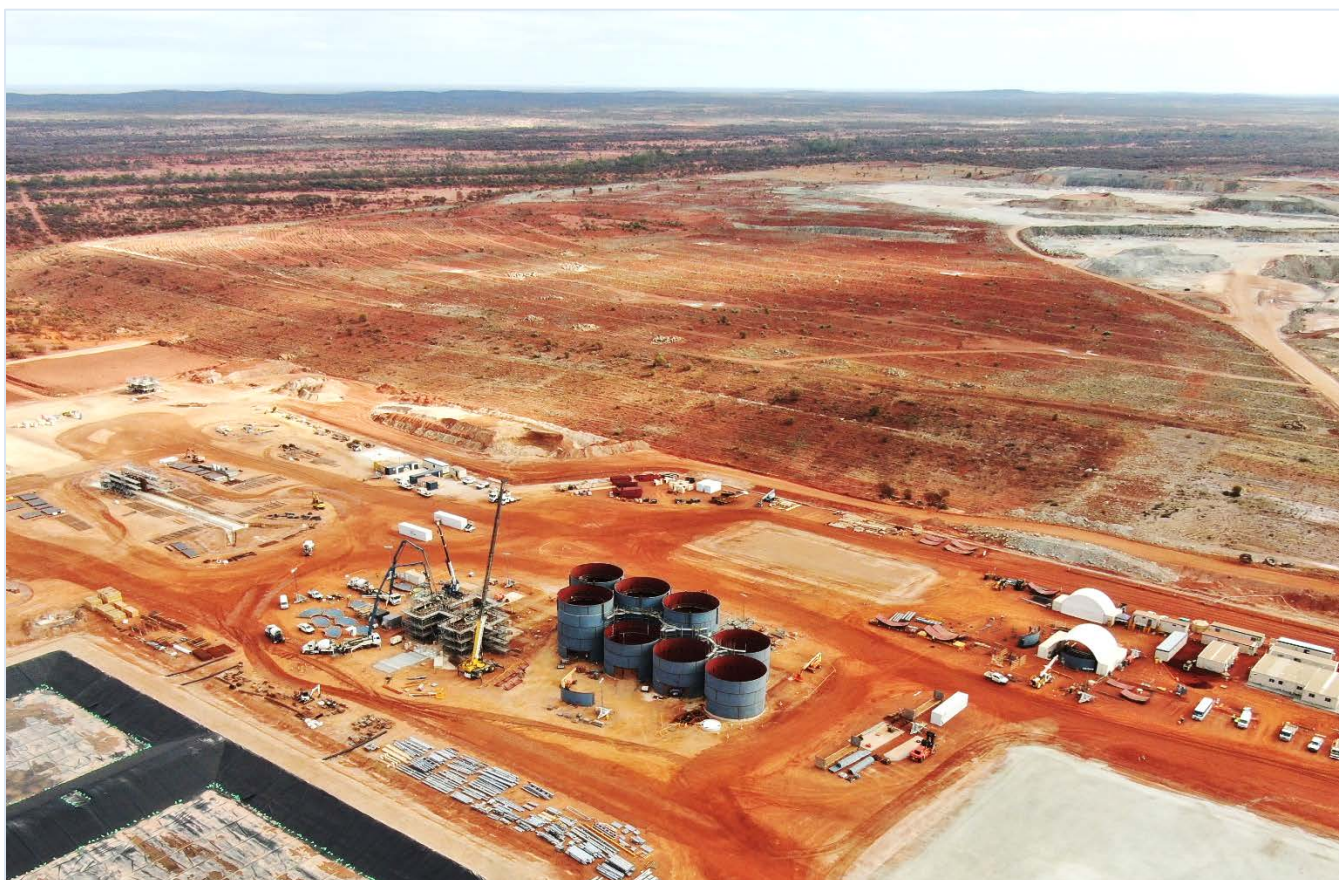
Figure 1: A two-day concrete pour of the mill plinths is being completed on 1 July 2021 and four of the eight CIL tanks are now at full height. Substantial steel deliveries are now on site, along with all major long-lead items in anticipation of the next key phase of steel-erection.
